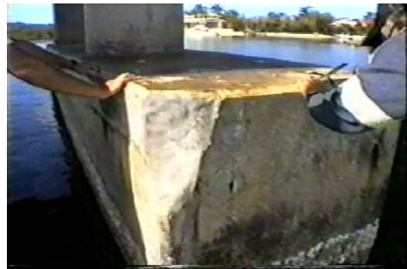
Photograph 3. Cracking and Spalling at the corners due to "Double diffusion".
