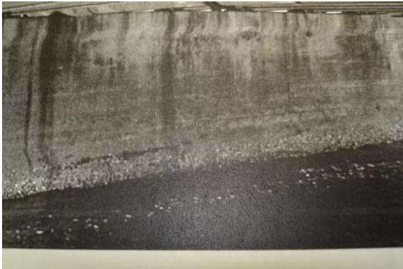
Photograph 6. Evidence of staining, rusting and delaminations on the sides of the pier
