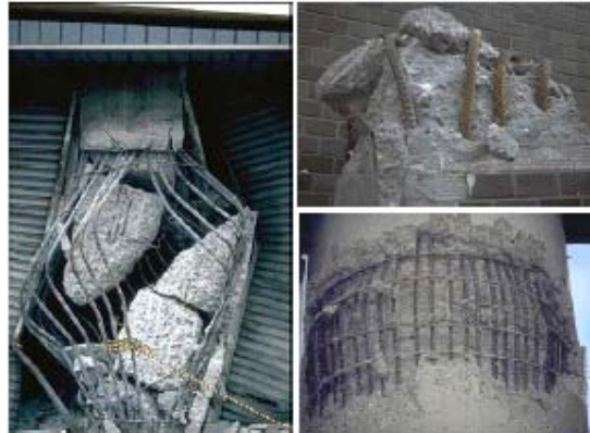
Figure 7-3: Column failures in Kobe 1995 earthquake (EQE 1995).
