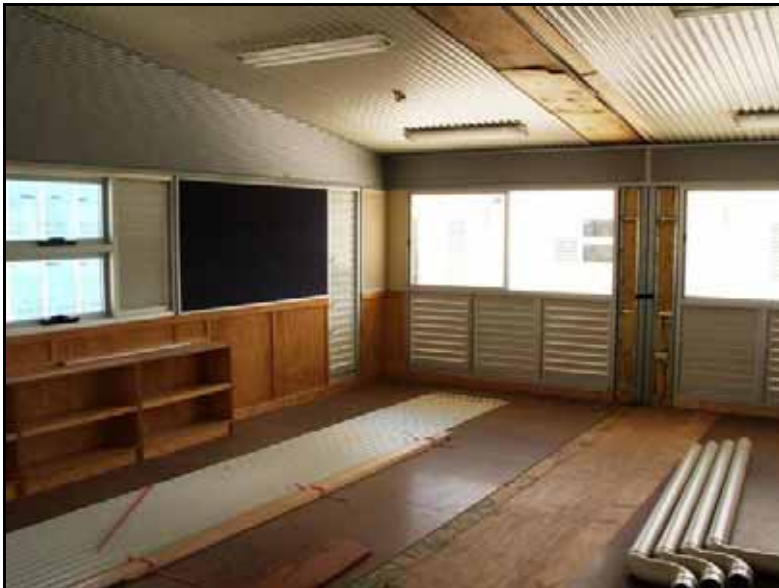
Figure 4.14: Completed classroom at factory showing cladding left off at module joints.
