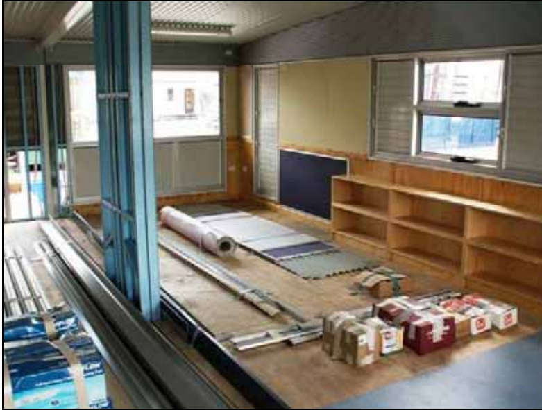
Figure 4.15: Completed classroom at factory showing cladding left off at module joints and transportation supports (blue steel).
