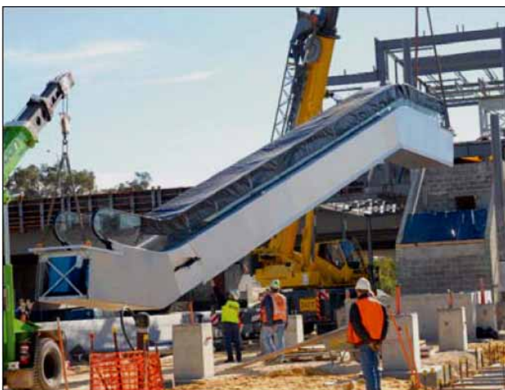
Figure 4.3: Bull Creek Station escalator being lifted into position (Source: New MetroRail 2006b)
