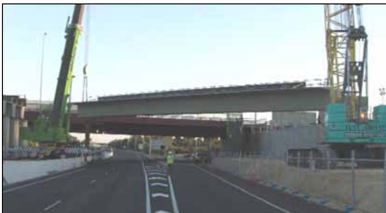
Figure 4.1: Leach Highway bridge T-Roffs being lifted into position (Source: New Metrorail 2006a)
