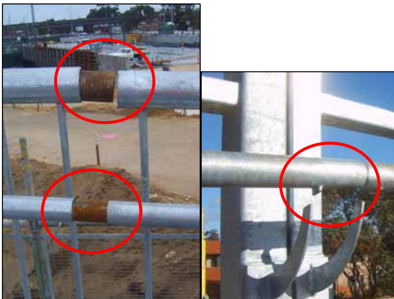
Figure 2.4: Balustrade on footbridge showing installation problems
