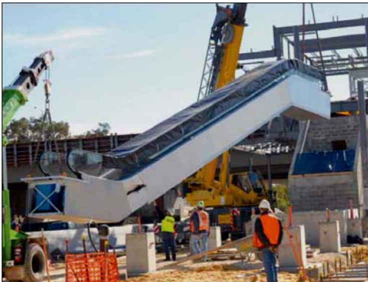
Figure 2.3: Bull Creek Station escalator being lifted into position (Source: New MetroRail 2006b)
