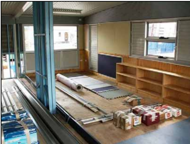
Figure 5.5: Completed classroom at factory showing cladding left off at module joints and transportation supports (blue steel).
