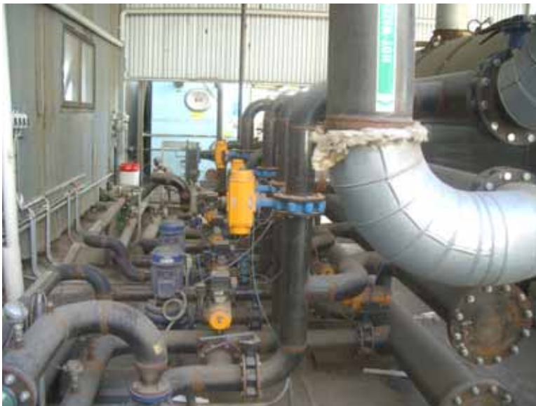
Figure 3.1: Boiler system used to accelerate curing of the moulded concrete.
