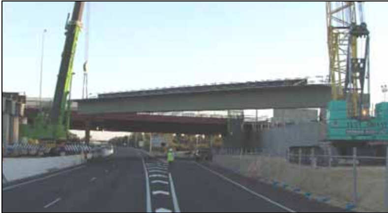
Figure 2.1: Leach Highway bridge T-Roffs being lifted into position (Source: New Metrorail 2006a)
