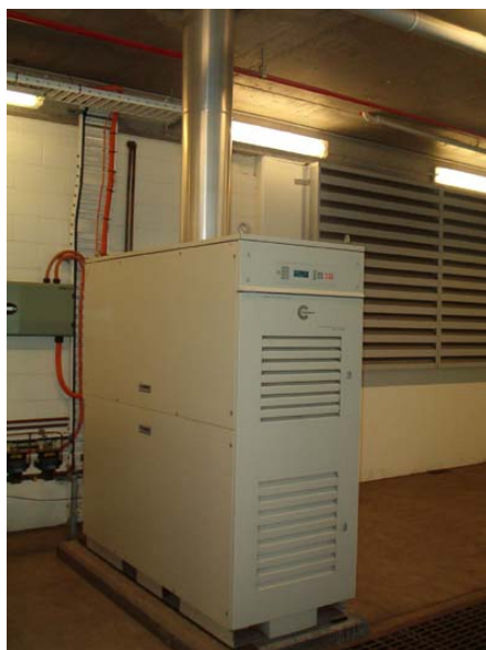
Figure 6.9 Typical micro co-generation turbine installed at the CSIRO Energy Centre
