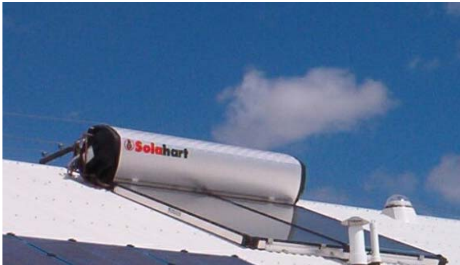
Figure 6.10 Solar hot water system installed at the Rockhampton research house
