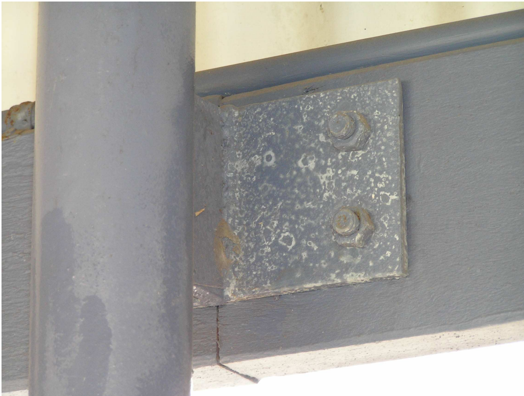
Figure 18 White corrosion product on painted steel brackets.
