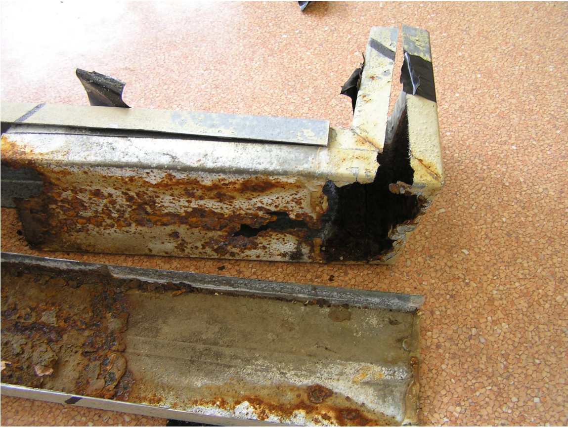
Figure A5, Top section of downpipe showing insert section that connects to gutter
