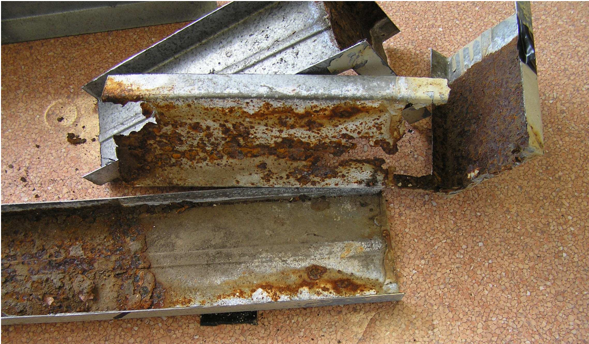
Figure A11, Insert used to connect the downpipe to the gutter, showing significant corrosion on lower surface.
