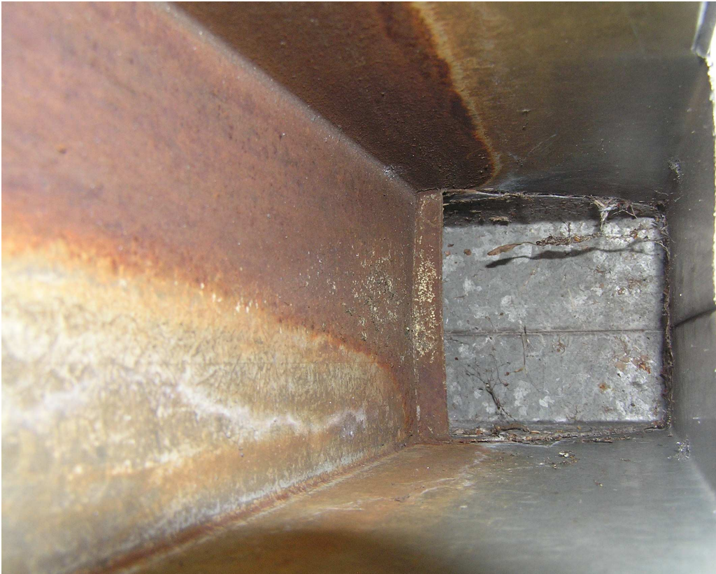
Figure A16, from inspection opening looking up to bend before gutter connection
