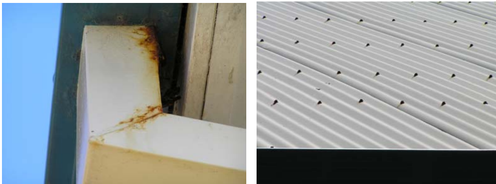
Figure 7.1 Examples of corrosion found in inspection of schools a) deterioration at joins of gutters, b) roof fasteners showing corrosion
