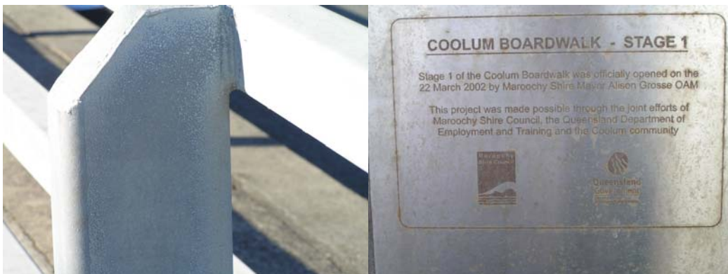
Figure 7.2 a) Bridge railing showing white corrosion product b) plaque showing “tea staining” from corrosion.
